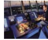
Multiple Control Displays
